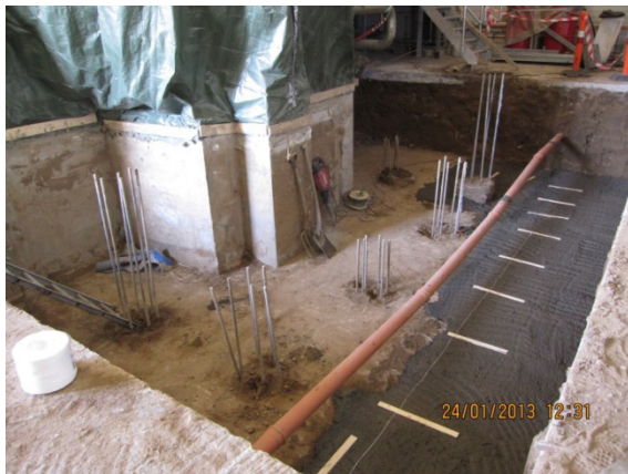
Figure 19: View on one side of the foundation after completion of the concrete piles.
