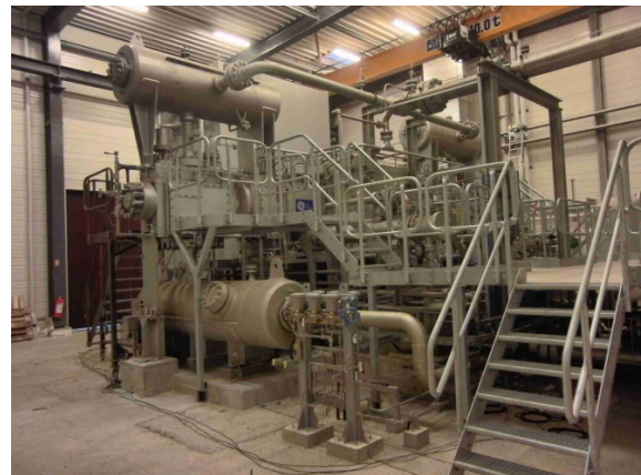
Figure 3: Compressor K-24 in the machine hall.
